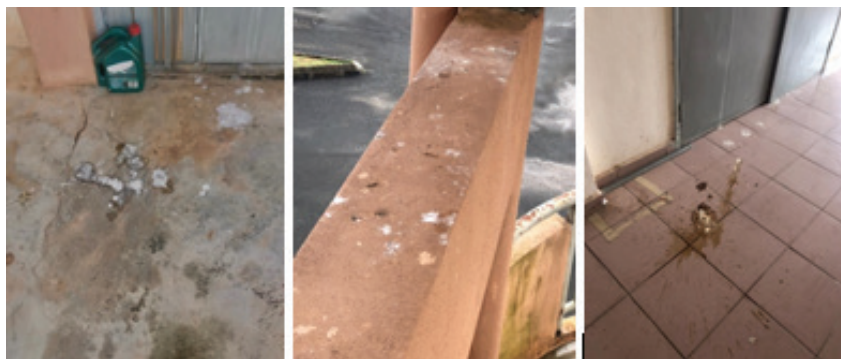
Figure 2: Bird Droppings Area in Various Sidewalk
